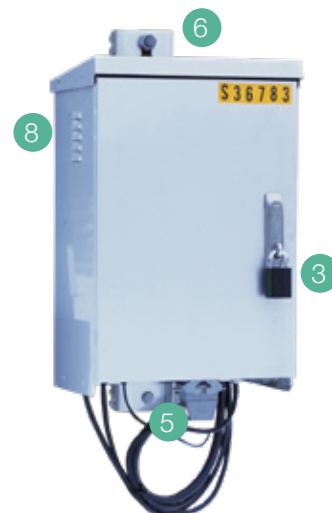
FTU recloser control cabinet
